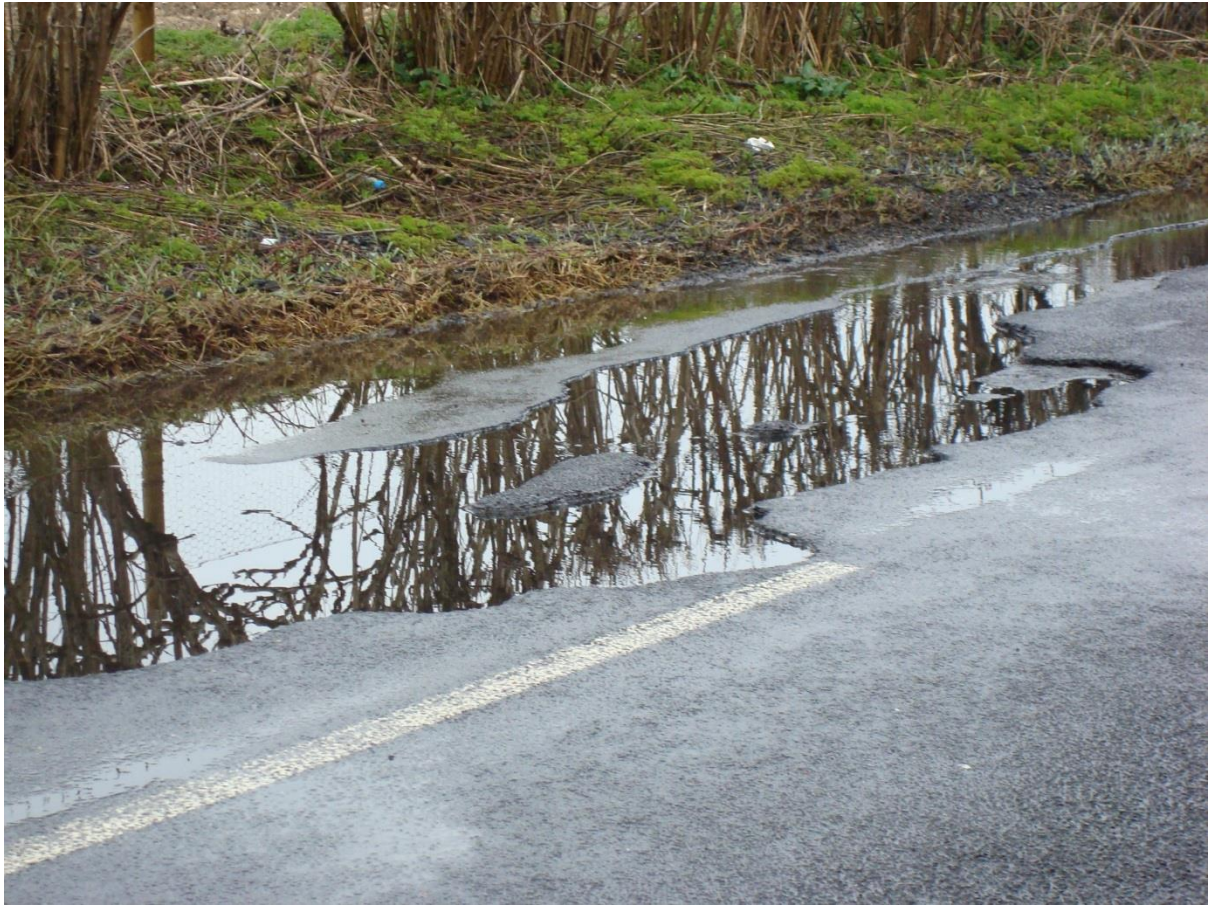
Bourne running westerly along North side of Ashford Road – tarmac surface destroyed out to white line in the middle of the road
